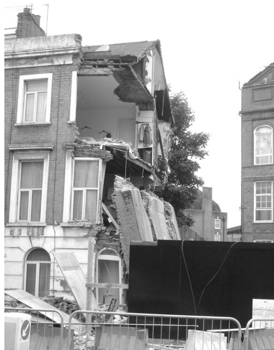
NO 101 BENWELL ROAD, REDUCED TO RUBBLE
