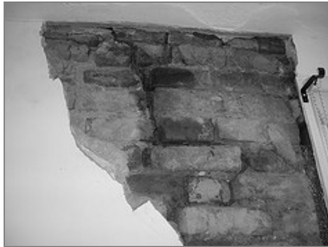
CRACK THOROUGHLY EXPOSED
